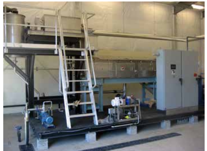
Class A Dewatering Skid Oroville, WA
