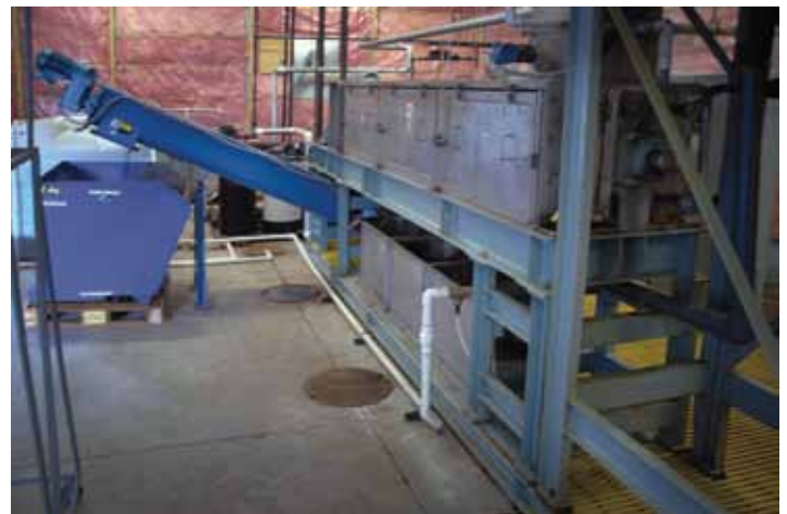
Class A Septage Dewatering Skid Big Fish Environmental Charlevoix, MI
