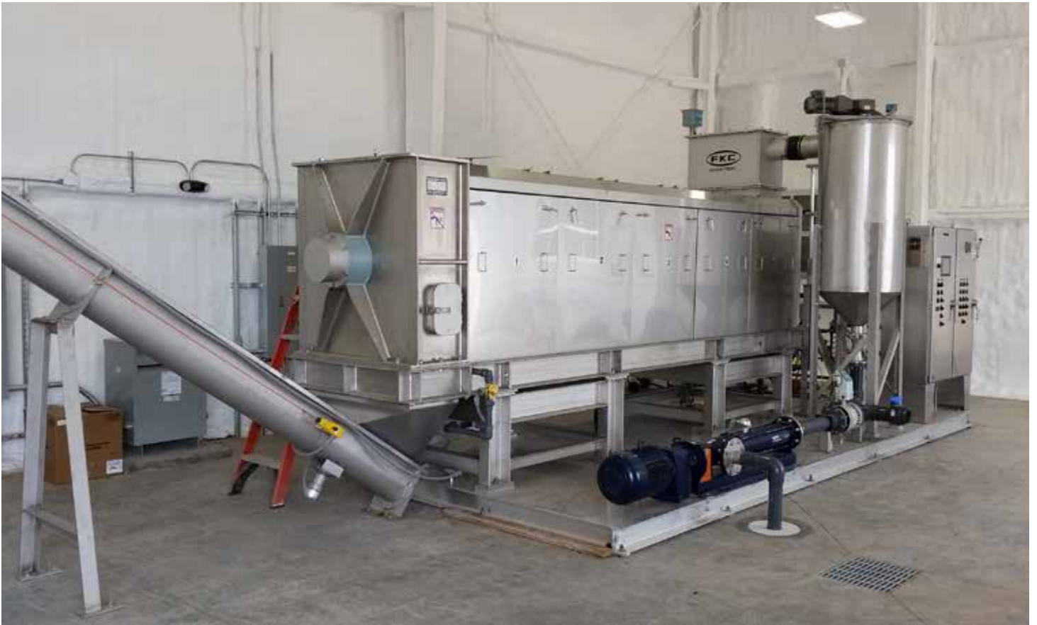
WTP Sludge Dewatering Skid
