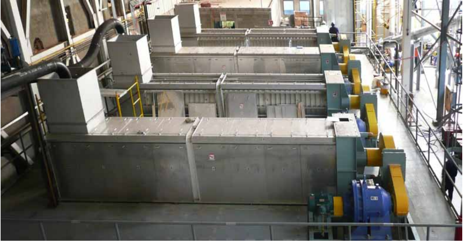
Four HX-1000 model screw presses installed at Grupo Modelo's Zacatecas, Mexico brewery.
