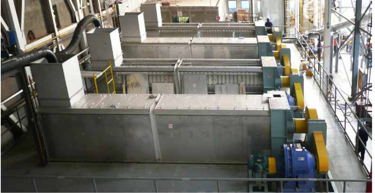
Four HX-1000 model screw presses installed at Grupo Modelo's Zacatecas, Mexico brewery.
