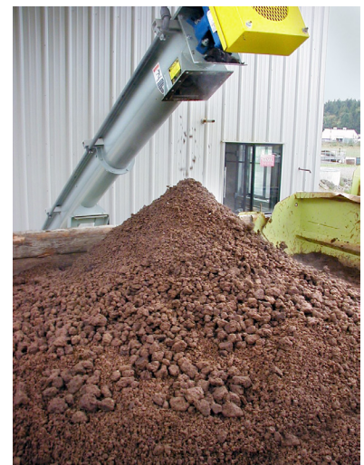
Dewatered and Pasteurized Biosolids from Sequim, WA FKC Class A Installation
